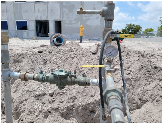
Photo No. 3 169 PSI recorded at 1:30 pm, two hours later.
