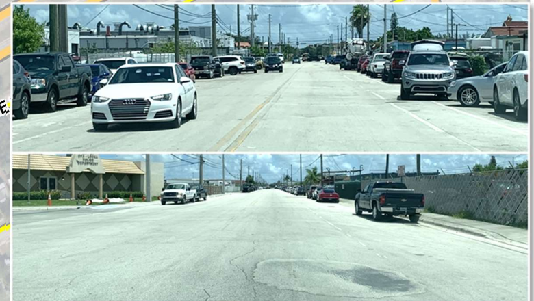
Ruts and Undulations in the Road Surface
