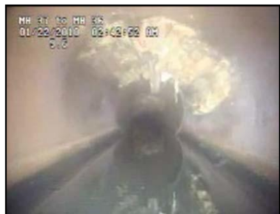
Gravity Sewer 1/22/2010 Downtown
