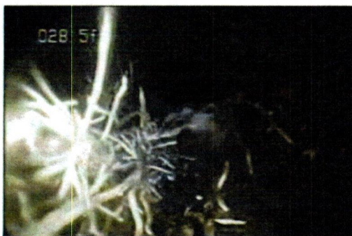
Roots in Sewer
